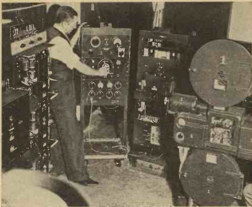
A corner of the projection room. One of the new multi-track sound heads is to be seen on the extreme right of the picture.
